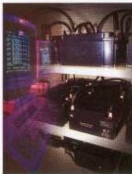
Battery Backup System
